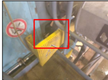
Fixed guard that does not designed in accordance with EN 13857:2008.
